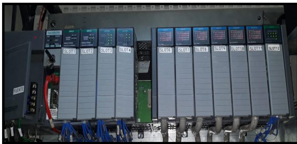
Figura. 1.7. PLC Allen Bradley 5000
