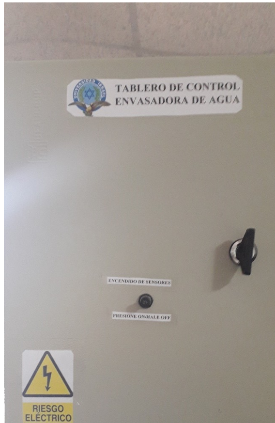
Fig. 8-2 Tablero de control
