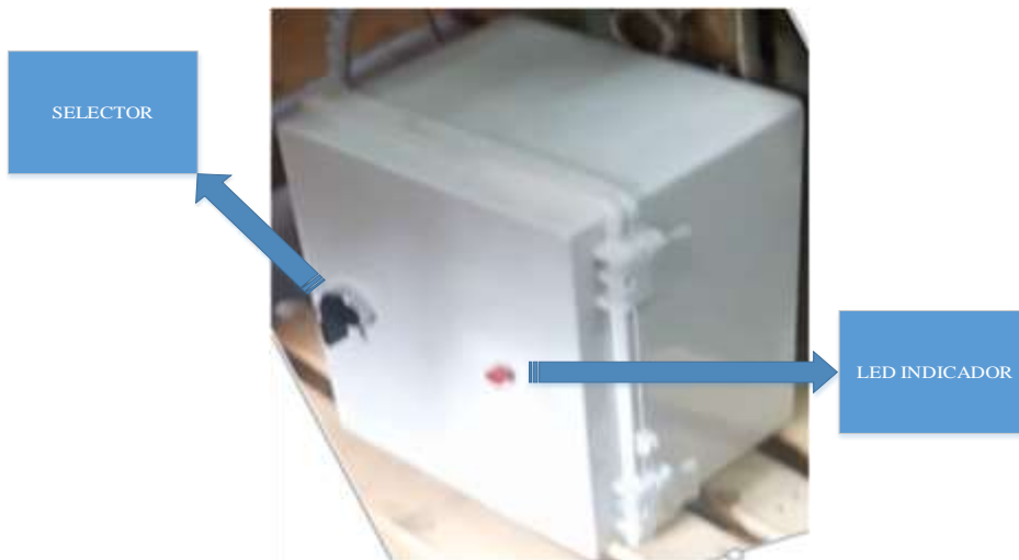
Figura. 4. 20. Tablero principal de control
