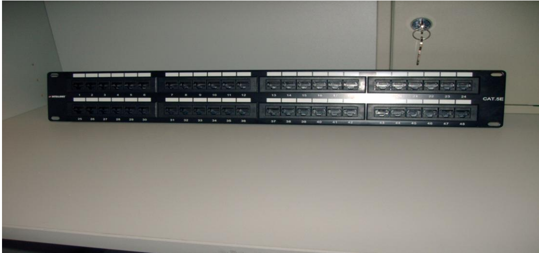
Figura 4.15. Patch Panel. Ruta
